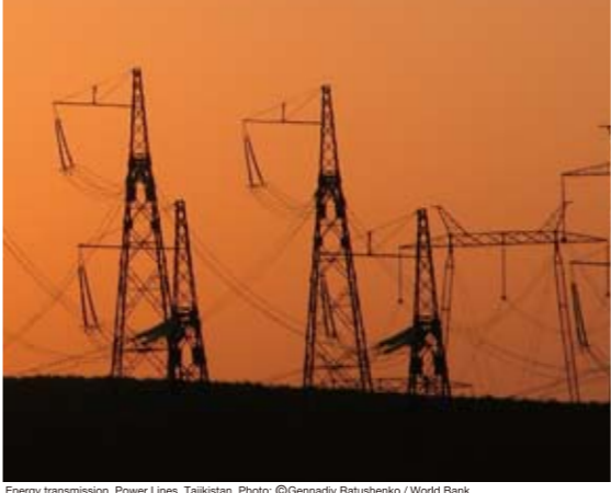
Energy transmission, Power Lines, Tajikistan, Photo: ©Gennady Ratushenko / World Bank
