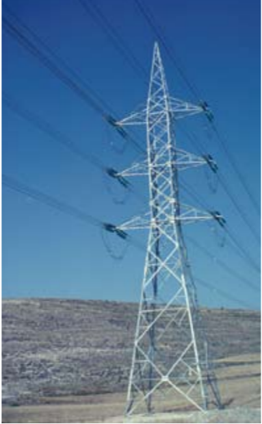
Power lines, Cyprus, Photo: ©Yusef Hadar / World Bank
